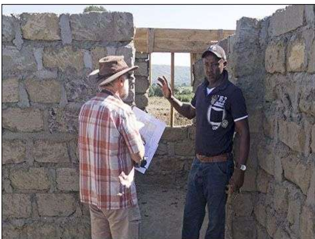
Nigel (left) one of our Trustees, with Ambrose (right) our local fundi (builder) discussing the plans for the new medical centre which is currently under construction. - 2013
